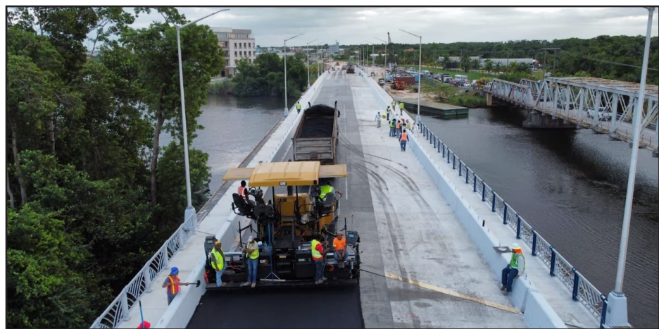
Pedestrian guard rails have not yet been installed on bridge
